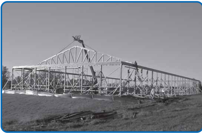
Work on the new covered outdoor arena at our Pegasus Farm chapter in Brewster, N.Y., is progressing on schedule for a late fall completion.
